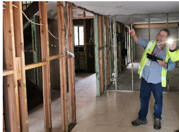
Photo Caption: 'Resilient Homes Fund staff conducting a site inspection on a flood affected property
