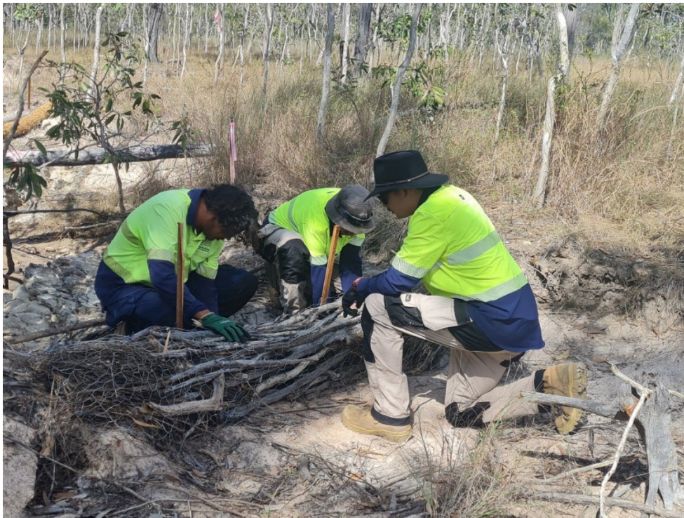
Photo Caption: Lewis Kyle, Gary Kyle and Tyreece Stanley from Three Big Rivers installing gully remediation stick weirs through the Townsville City Council Reef Assist 2.0 project
